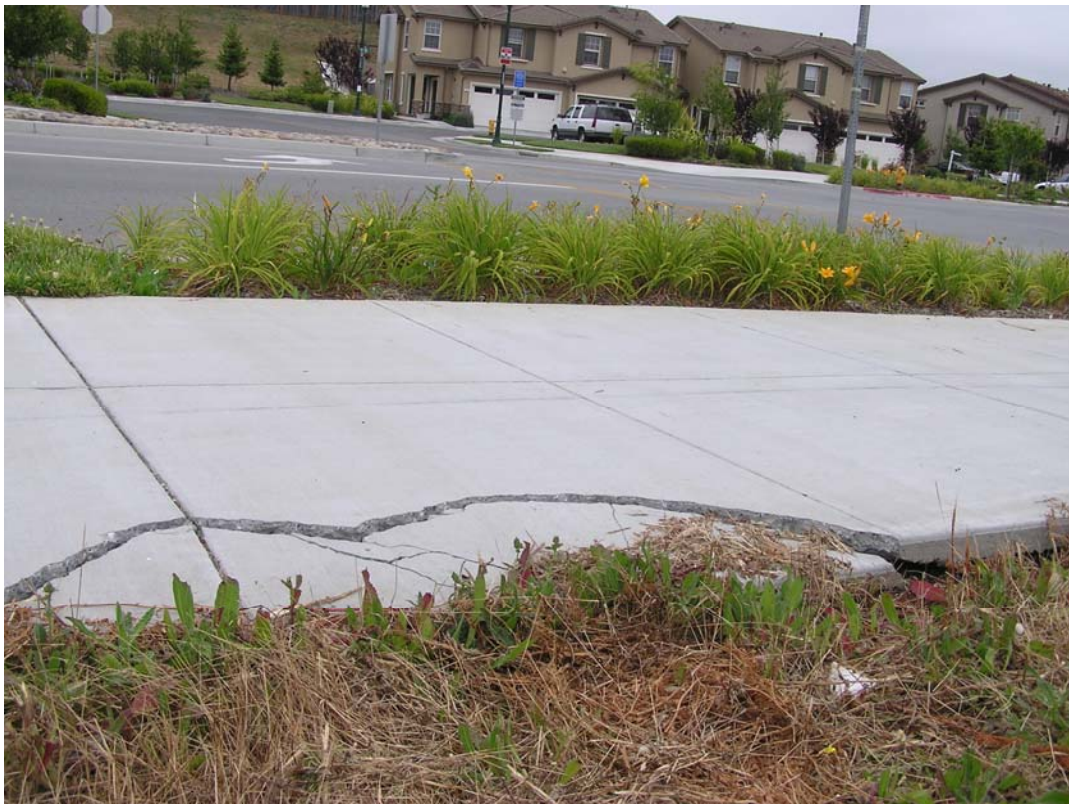
Figure 6. Crack in new sidewalk.
