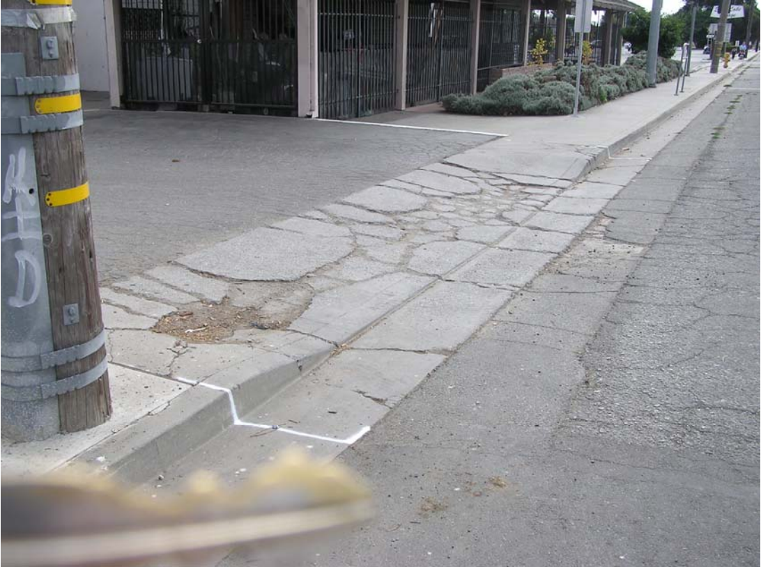
Figure 2. Large cracks in driveway.
