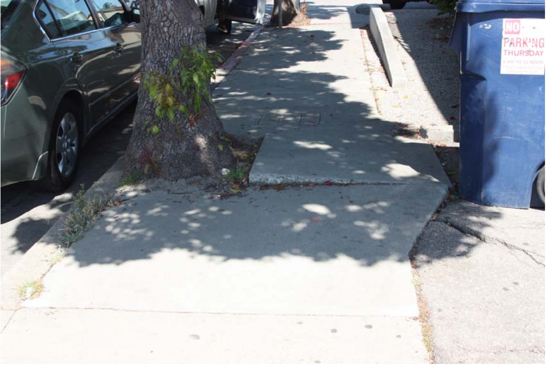
Figure 1. Sidewalk uplift due to tree roots.
