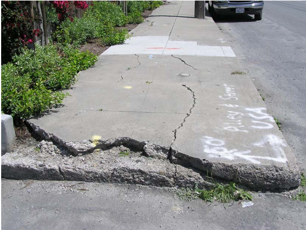
Figure 5. Deterioration of sidewalk curb.
