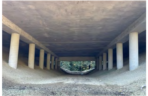
Highway 17 Wildlife Crossing
