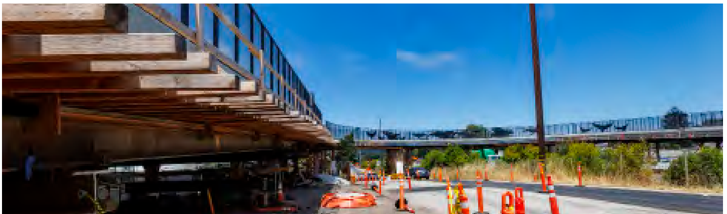
Bicycle/pedestrian bridge construction over Highway 1 at Chanticleer Avenue (photo by Kevin Painchaud)
