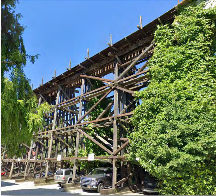
Timber substructure for Segments “B” and “D” require total replacement
