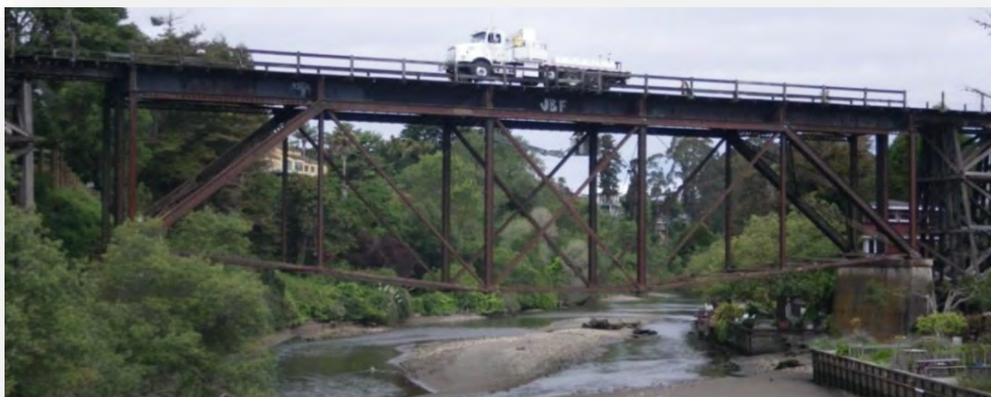
Concrete piers for truss are located within ordinary high water of stream channel
