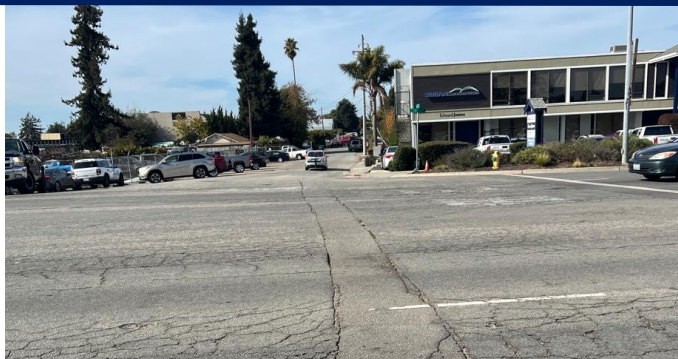
Old Utility Trench Repairs and Faded Striping
