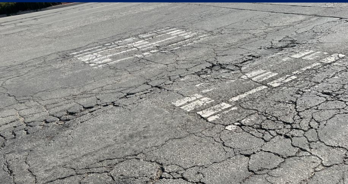
Depressions and Uneven Pavement
