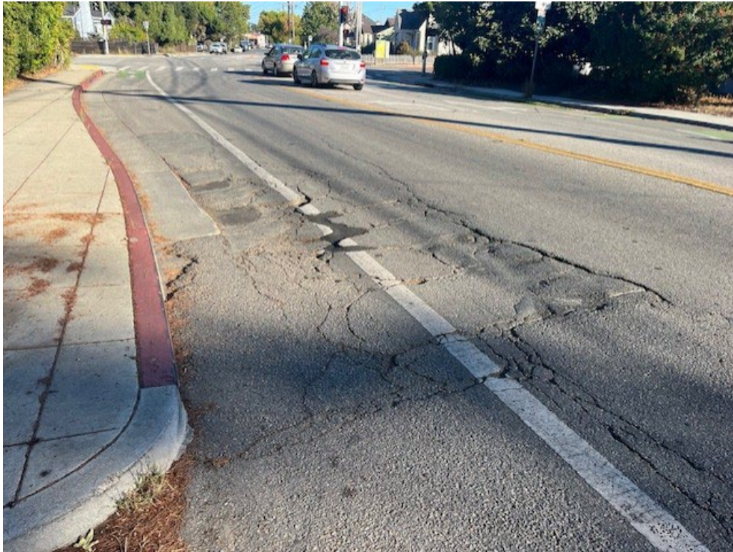
Figure 5 Example deteriorated pavement condition. The user experience for people biking, driving, or taking transit is very bumpy here due to the pavement.
