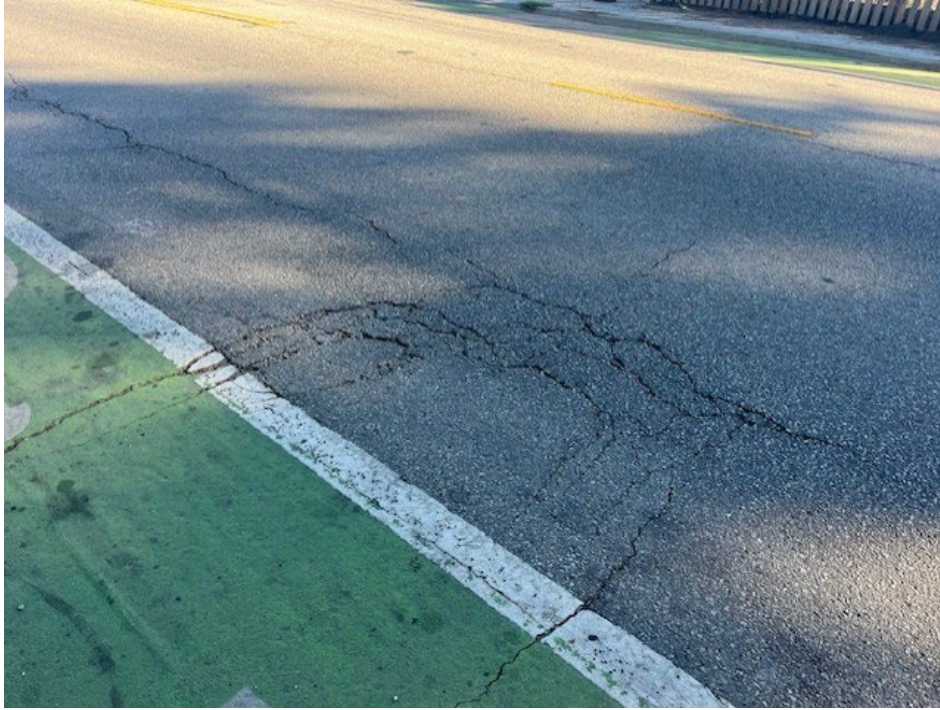
Figure 4 Example pavement condition
