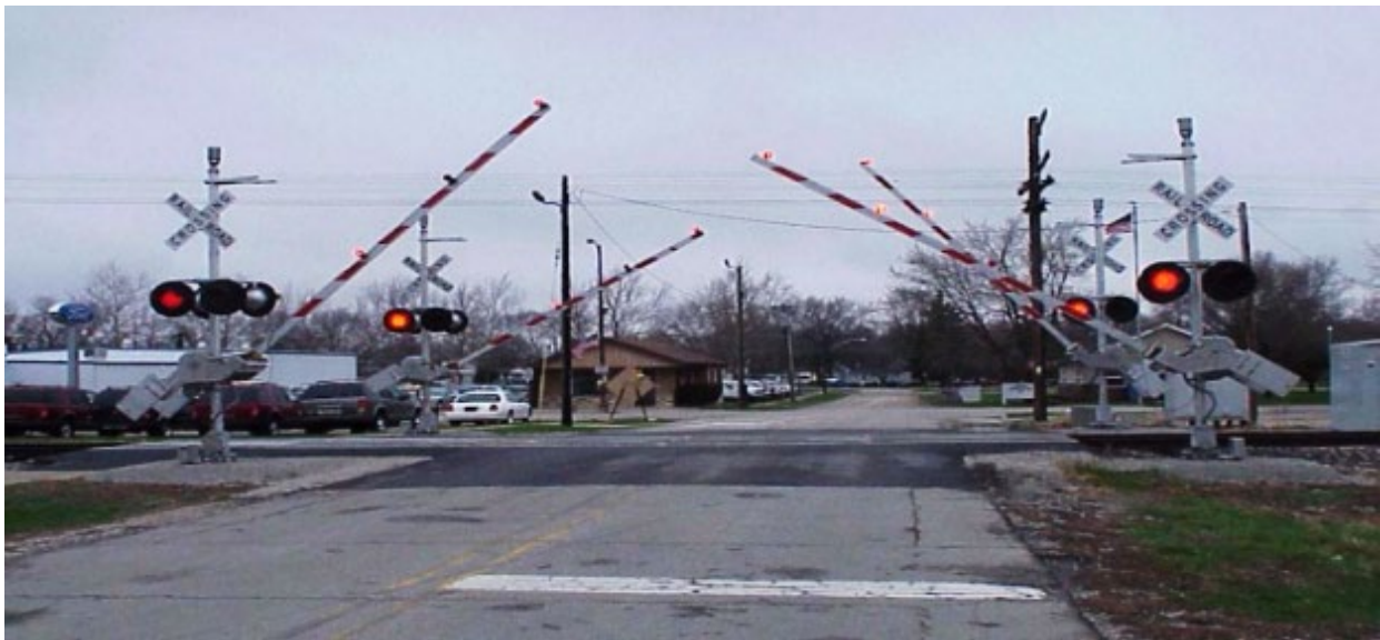
Figure 8.1 Example Four-Quadrant Grade Crossing System
