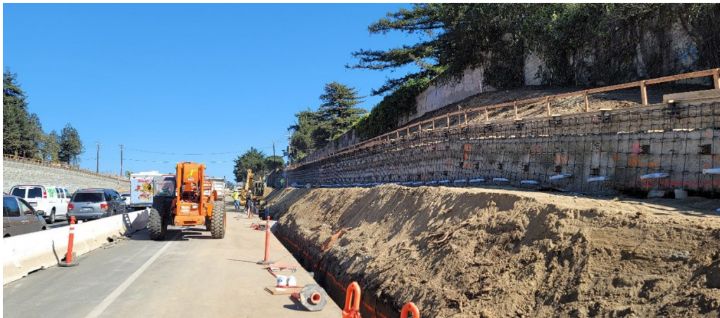
Construction on the Highway 1 auxiliary lane and bus-on-shoulder project between Bay Avenue/Porter Street and State Park Drive
