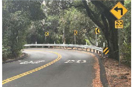
Pavement rehabilitation on Bean Creek Road (before & after), City of Scotts Valley
