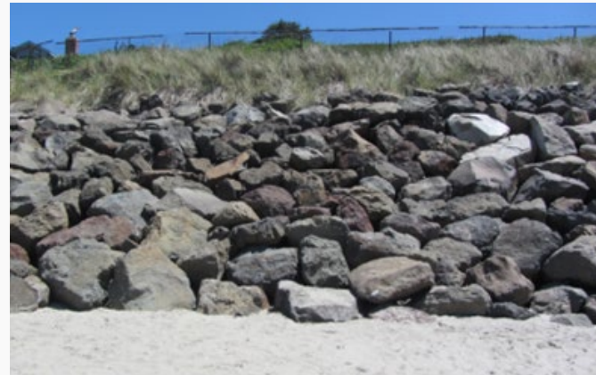
Rock Slope Protection
