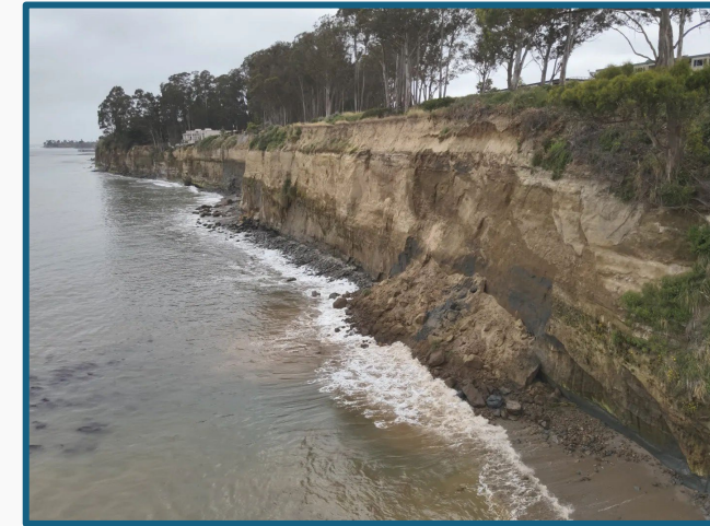
Erosion at Capitola Bluff Image Source: santacruzsentinel.com
